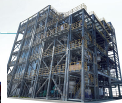
BDO Reaction Skid-Mounted Equipment 2025 Jiangsu, China
